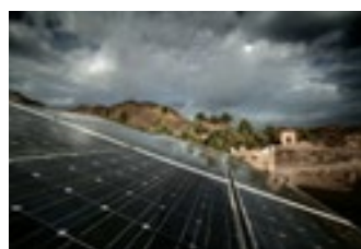
Photovoltaic power plant in Morocco.
