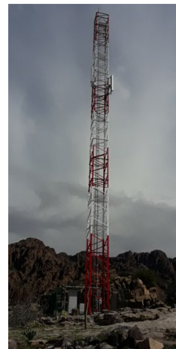
Image of the works developed by Abengoa in Morocco for Orange.
