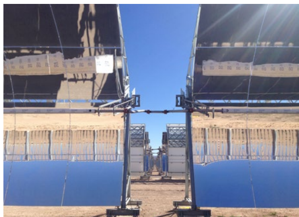
Parabolic trough collectors of the Agua Prieta II solar-gas hybrid plant, of which Abengoa has been responsible for the 14 MW of solar power.
