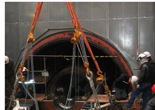
Major inspection in the gas turbines of the ISCC Plant Ain Beni Mathar (Morocco).
