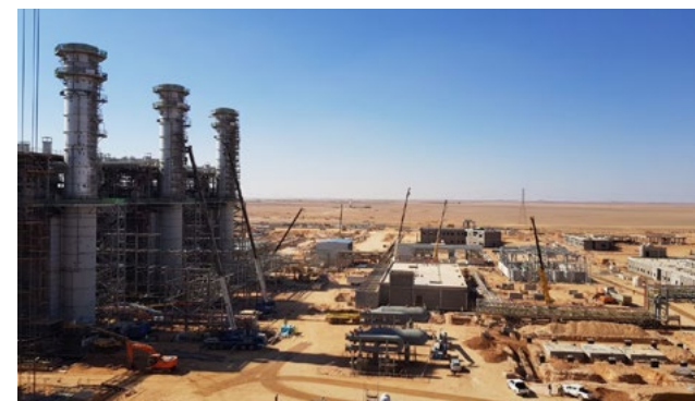
Image of the works that Abengoa is developing in Saudi Arabia in Waad Al Shamal plant.
