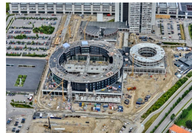
Abengoa develops the electromechanical facilities of a hospital in Herlev (Denmark).
