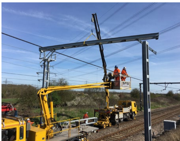
Abengoa carries out catenary works on different lines in the United Kingdom.
