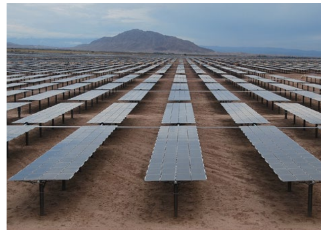
Photovoltaic plant developed by Abengoa in California.
