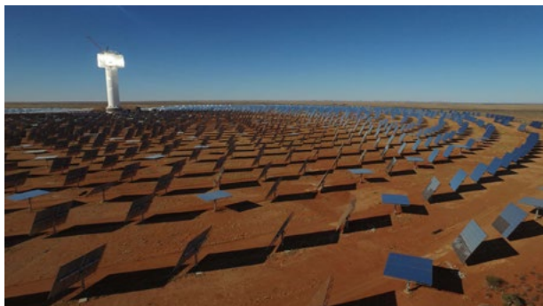
Khi Solar One has a capacity of 50 MW and two hours of storage.
