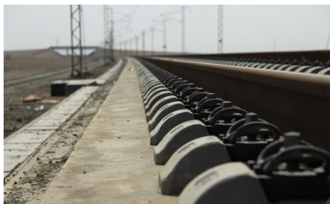
The broken track project allows rapid detection of track breaks.
