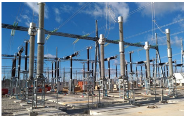
400/22kV substation that Abengoa is developing at ITER.
