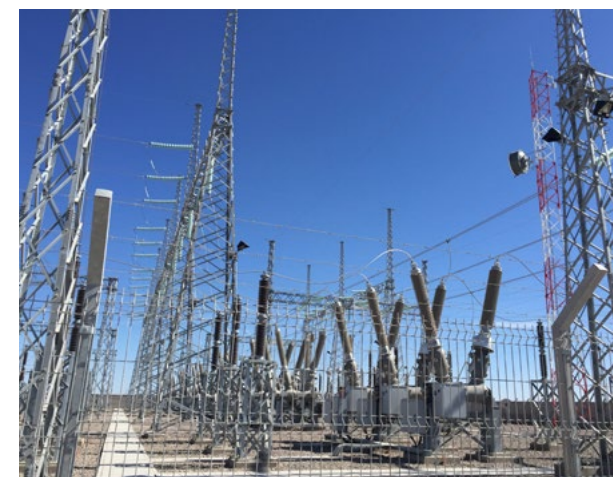
Switching station of the Atacama I project, of the Cerro Dominador solar complex.
