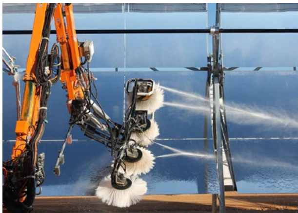
Vehicle for cleaning the parabolic troughs.
