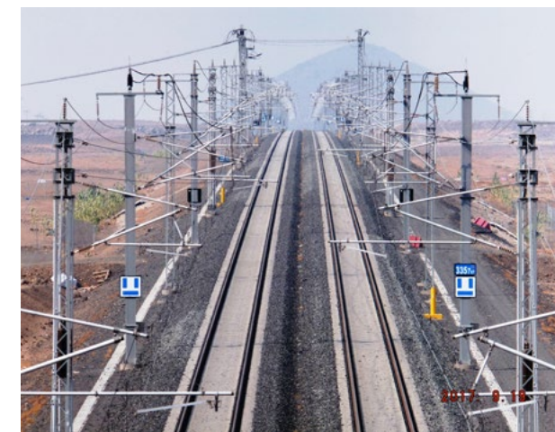
Abengoa takes part in the construction of the high-speed line between the cities of Mecca and Medina.
